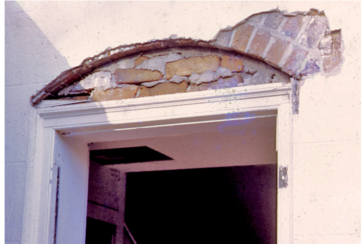
This photo shows how the original poorly fired brick had been protected by an application of stucco early in the life of the house.
