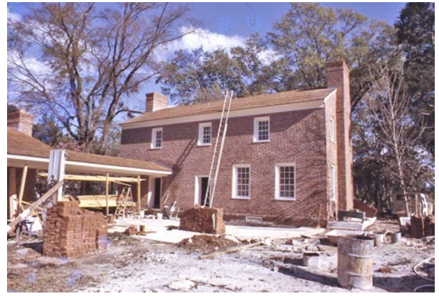
The original detached kitchen was recreated and connected to the house by a covered walkway.
