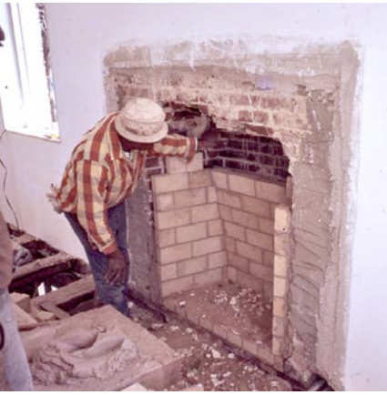
Specially trained and skilled brick masons were a must for this job.
