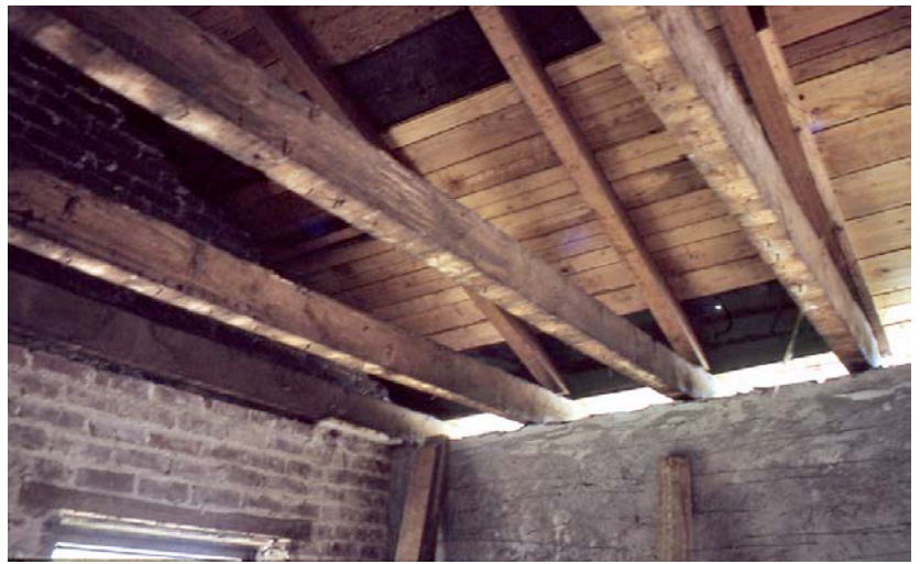
Rough hewn 1820s-era rafters were also discovered as the house was carefully taken apart during the initial stages of the restoration process.
