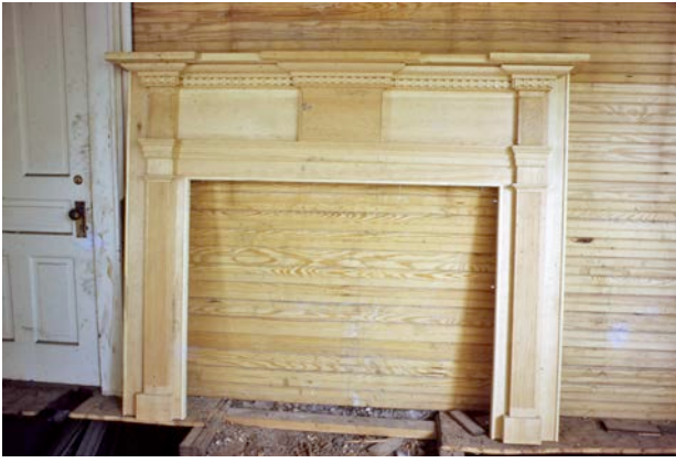
This mantelpiece was original to the house. It was sent away to be stripped and returned for reinstallation.
