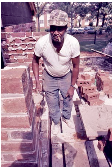
An experienced historic preservation crew brought with it the craftsmanship needed for good results.
