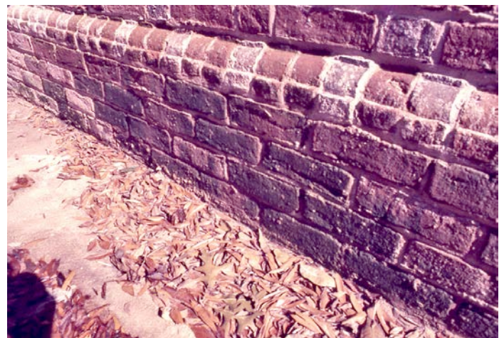
A new border of regular and "bullnose" brick gave the foundation of the King House an attractive and authentic masonry accent.
