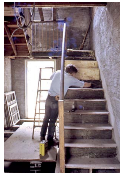
The original staircase was repaired, reinforced, and refinished for an attractive and safe appearance
