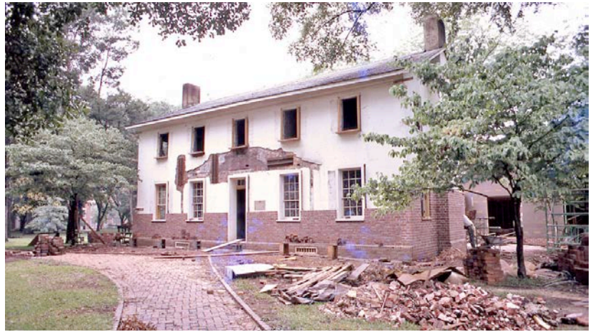
A layer of new brick was laid over the old stucco and original brick veneer.
