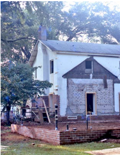
The original profile of the house emerges after removal of the addition.
