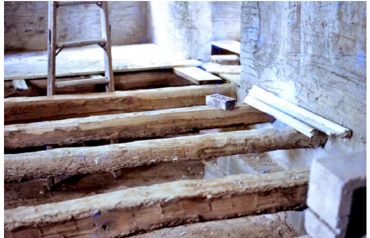
Hand hewn timbers had been used as original floor joists. They were discovered still intact and usable in the restoration.
