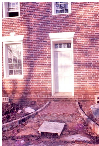
Employing Federal period brick patterns lent a sense of authenticity to the restoration
